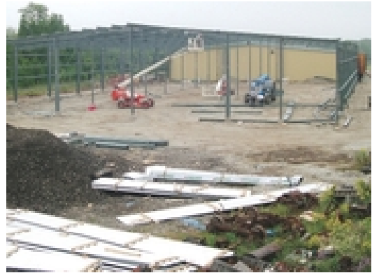
Construction has begun on the Sir Adam Beck Centre, which will provide storage for the Halton County Radial Railway Museum.
