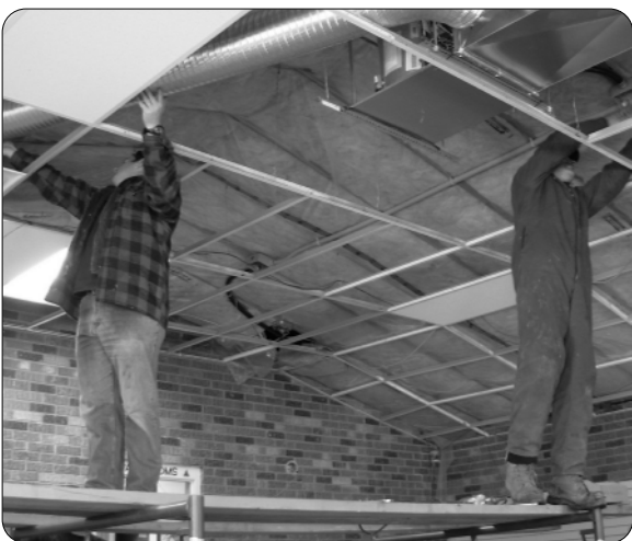
Members Tom Twigge-Molecey and Ian Smith installing the new furnace in the Gift Shop
